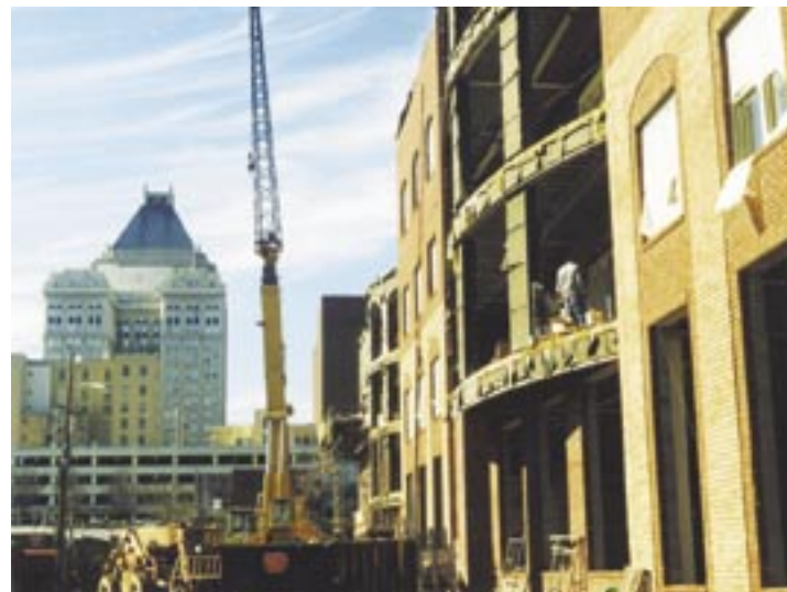
Governor's Court Condominiums under construction: another example of progress in downtown Greensboro.
